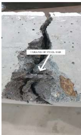
Figure 11. Failure of steel bar.
